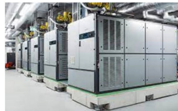
Combined heat & power system implementation
